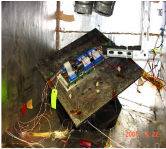
Fig. 1. Unit on the skewed ESS system
